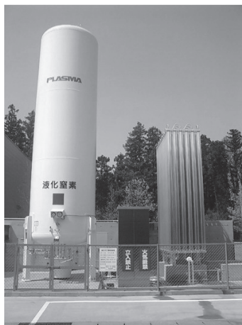
Fig. 23 Storage tank of liquefied nitrogen and gas pressure boosting system
